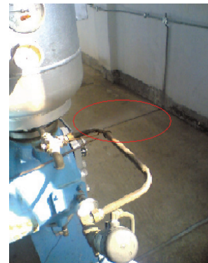
Fig. 8 Example of detected leakage spot
