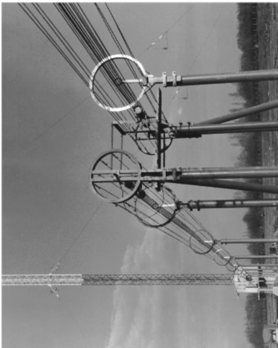
Picture 1. MF broadcast antenna of Radio Podgorica. The antenna feeder line is in front plane. The building-ground height is about 185 m, and elevated antenna base height is 3.3 m. The mast has four levels of stays which are arranged in the three vertical planes symmetrically placed at 120^\circ angles. The antenna operating frequency is 882 kHz, and unmodulated carrier power is 600 kW.
