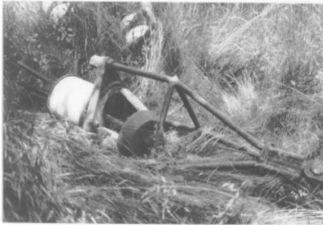
Fig. 2. An old ceramic stay insulator damaged by RF arcing.
