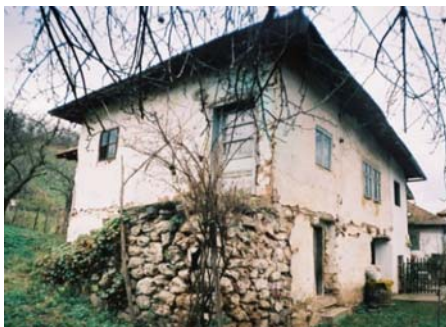
Fig. 7. Old house (with inadequate addition)
