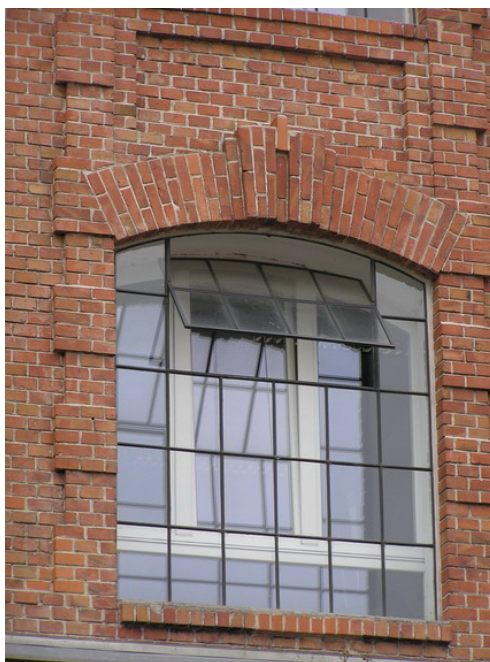
Fig. 6. Renewal of facades: the external walls are cleaned and repaired if necessary, new window is placed behind the original one.
