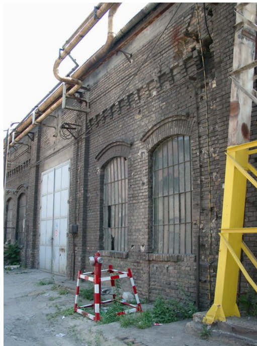
Fig. 1. Industrial building in poor condition: various building failures can be observed
