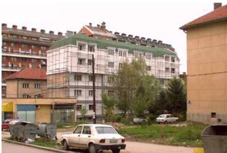
Fig. 8. Appearance of the building after the addition of a storey and loft viewed from the southwest side.
